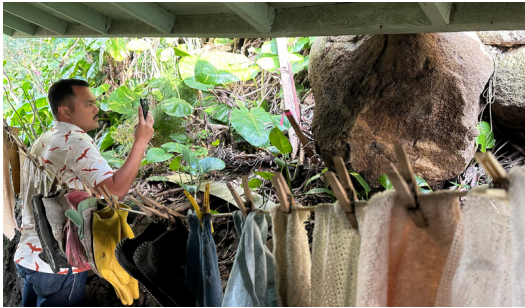
Inspecting a boulder at a home on Anu'u Place in Kalihi Valley, which has been lodged behind a neighbor's home between a retaining wall and a roofline.
